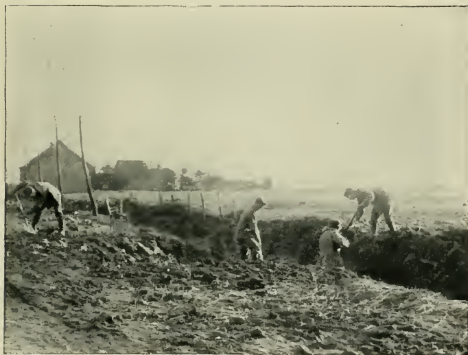
A SHELL CRATER IN THE ROAD IS BEING FILLED IN BY ENGINEERS
