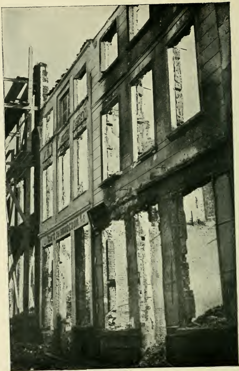
SOME HOUSES ONLY HAVE THE WALLS LEFT STANDING
